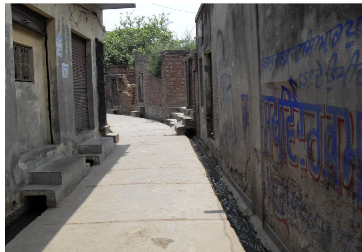
OPEN DRAINS ON BOTH SIDE OF STREET
