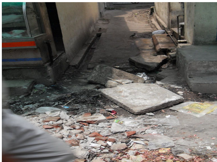
OPEN DRAIN, NO SEWERAGE
